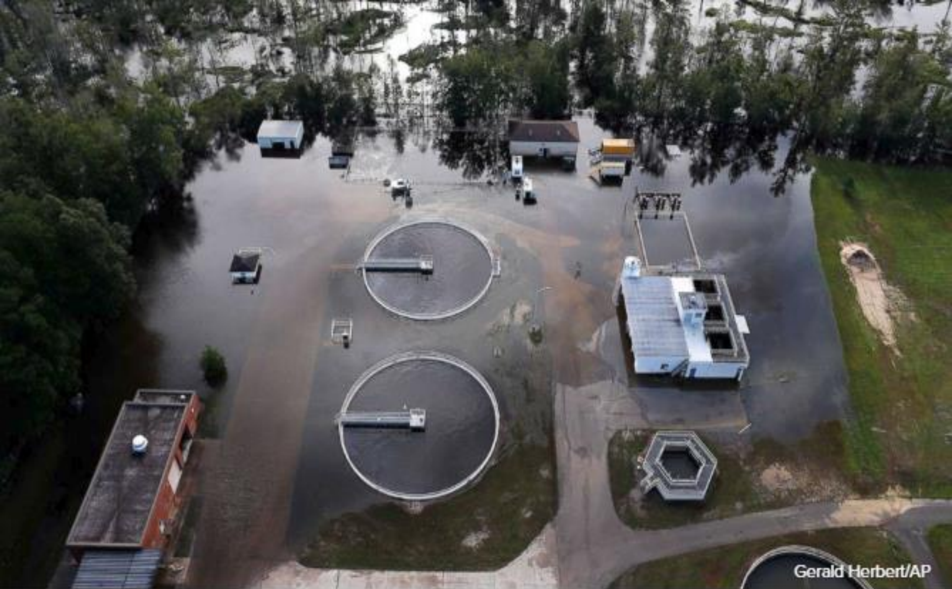
A wastewater treatment plant is inundated from floodwaters in the aftermath of Hurricane Florence in Marion, S.C., Sept. 17, 2018.
